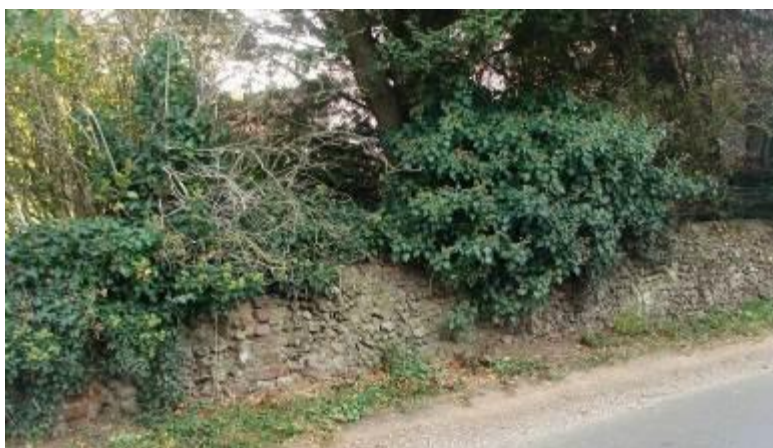
Picture 15: Wall at Gravesend Farm that would benefit from repair work and removal of ivy
